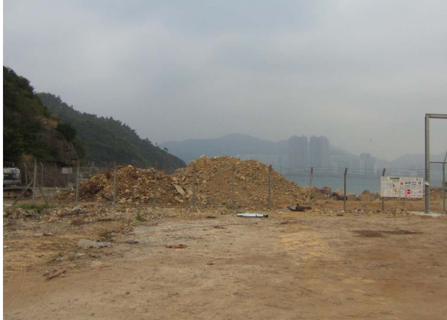
Photo 1 –Stockpiles of the excavated materials were observed to be exposed.
