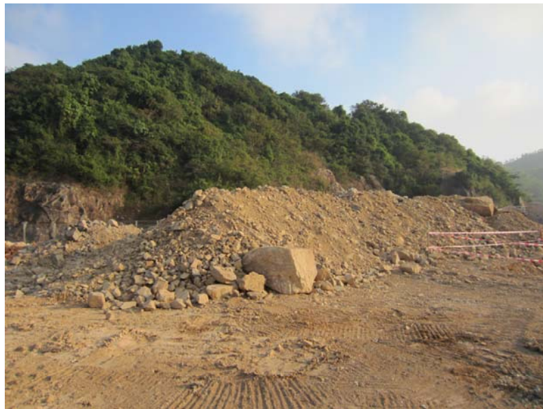
Photo 2 - Stockpiles of the excavated materials were observed to be exposed.
